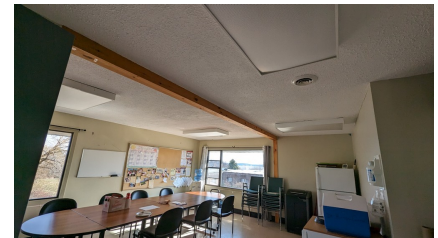
Figure 67: Type A1 - surface mounted fixtures assumed to have T8 lamps
