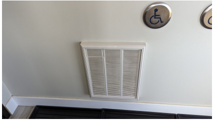
Figure 35: Electric heater at entrance to dentist office
