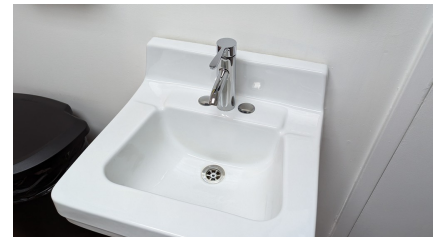
Figure 108: Examination room sink
