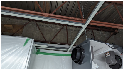
Figure 10: No insulation on foundation wall
