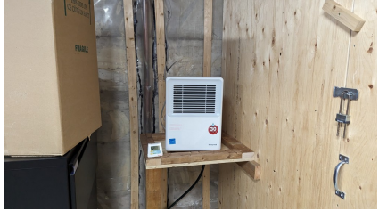
Figure 53: Portable dehumidifier in storage room-2
