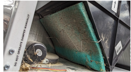
Figure 40: HRV1 dirty filter
