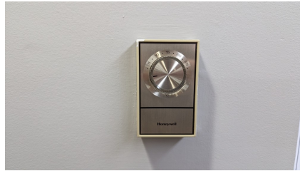
Figure 57: Thermostat for an electric heater in the waiting room
