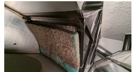
Figure 34: Dirty filter on HRV4
