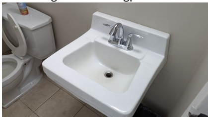
Figure 109: Hand faucet in the basement
