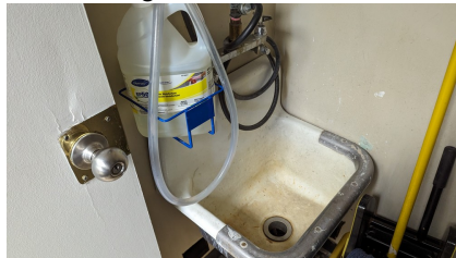
Figure 119: Sob sink in the basement
