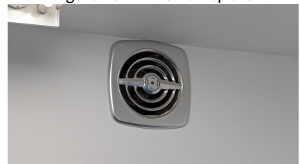
Figure 49: Men's washroom exhaust
