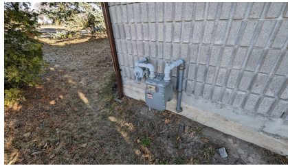
Figure 124: Natural gas meter
