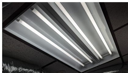
Figure 69: Type A3 - retrofitted with LED lamps
