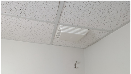
Figure 38: Exhaust fan in dentist area washroom
