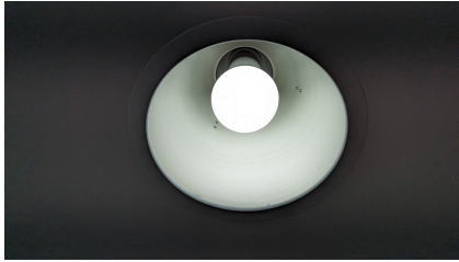
Figure 74: Type C1 - Vestibule lighting with LED lamp
