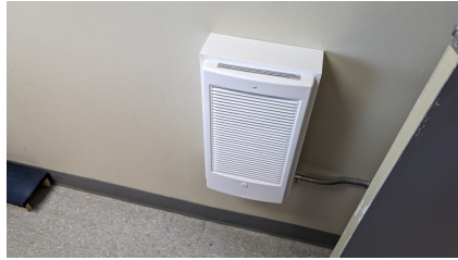
Figure 36: Electric heater in room 240
