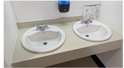
Figure 117: Men's washroom faucets
