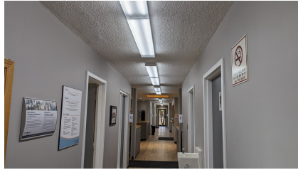
Figure 75: Type C2 - replaced 1x4 surface mounted fixtures with LED lamps
