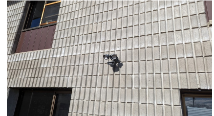
Figure 64: Flood lights with integrated motion sensor
