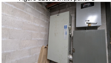
Figure 129: Main switch - 600A
