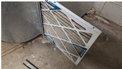
Figure 23: AC3 dirty filter
