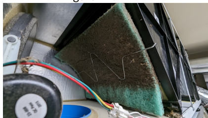
Figure 45: HRV3 dirty filter
