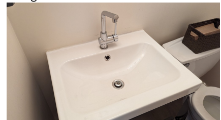
Figure 111: Handwashing faucet in rm 105
