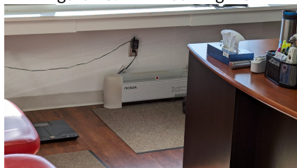
Figure 51: Plug in electric heater in an office
