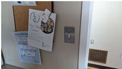
Figure 65: Manual switch in room 243
