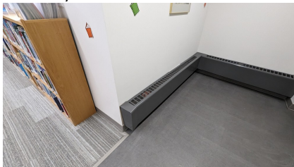
Figure 33: Hydronic baseboard heating
