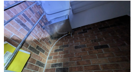
Figure 32: Elevator exhaust fan
