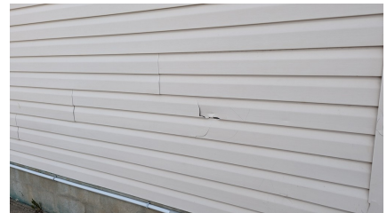
Figure 8: Damaged vinyl siding on the east elevation
