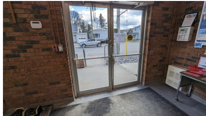
Figure 10: Front entrance with gap between doors
