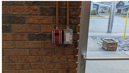
Figure 53: Control switch in the lobby
