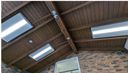
Figure 52: Ceiling-mounted occupancy sensor in the lobby
