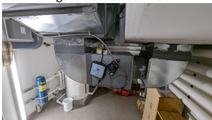
Figure 39: System bypass damper
