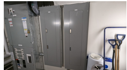
Figure 82: Panel A and B - both labelled incorrectly
