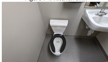
Figure 77: Toilet in WR 108
