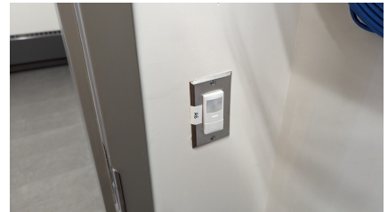
Figure 54: Light switch with occupancy sensor
