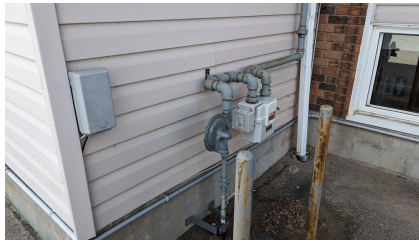
Figure 79: Natural gas meter
