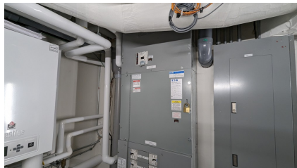
Figure 80: 400A main breaker
