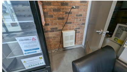
Figure 31: Electric forced flow heater in the lobby
