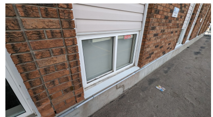
Figure 17: Vinyl window framing in poor condition
