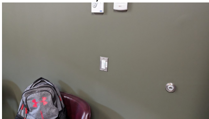
Figure 55: Light switch with dimmer in an office
