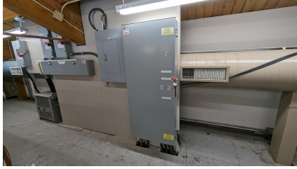
Figure 87: Transfer switch - radio station
