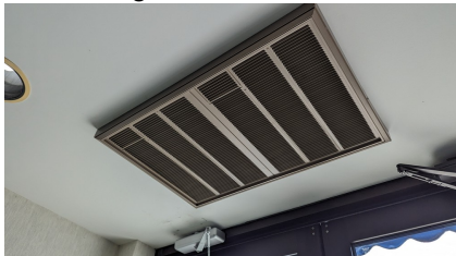
Figure 27: Heater in vestibule to radio
