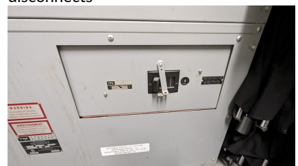
Figure 83: Main disconnect - building
