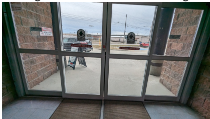
Figure 7: Gap in front entrance to the hall
