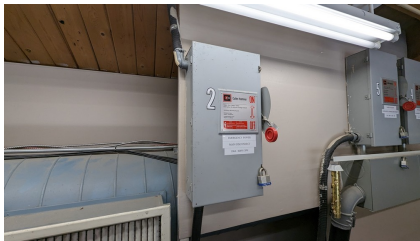
Figure 75: 100A emergency power disconnect
