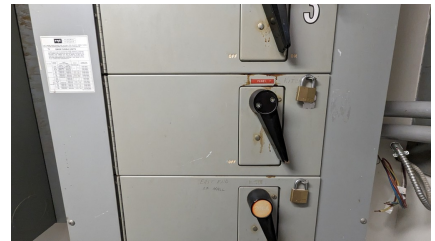
Figure 77: 200A disconnect for Panel C
