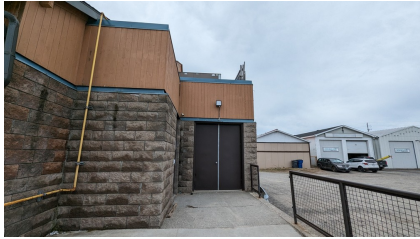
Figure 10: Hollow metal doors
