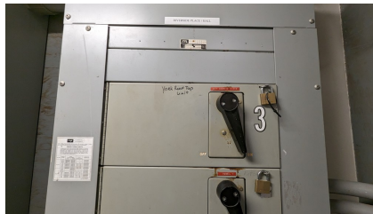
Figure 76: 200A disconnect for AC1
