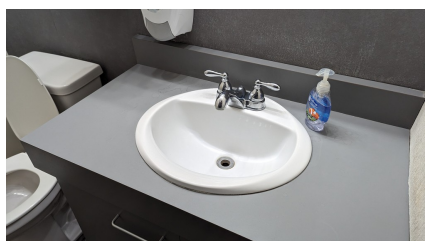
Figure 63: Faucet in radio washroom
