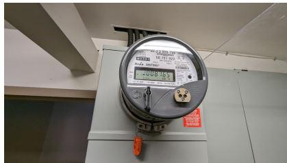
Figure 72: Electricity meter - radio
