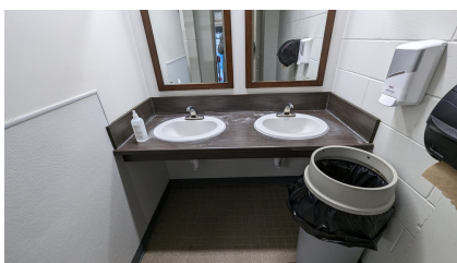
Figure 64: Handwashing faucets in men's washroom
