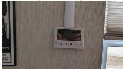
Figure 28: HRV controller in room 27
