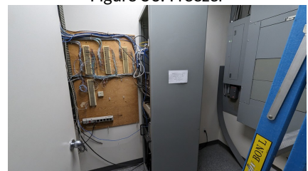
Figure 59: IT equipment in room 39
