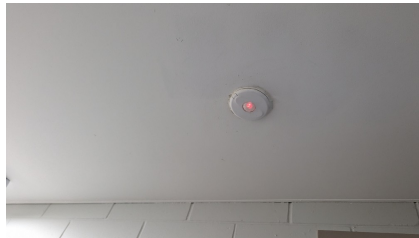
Figure 38: Occupancy sensor in the men's washroom
