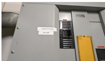
Figure 82: Main disconnect - radio
