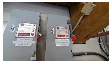
Figure 80: Emergency power disconnects
