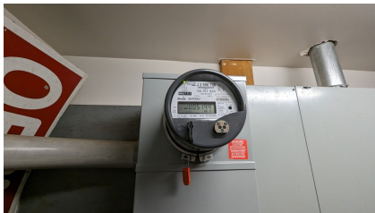
Figure 71: Electricity meter - hall
