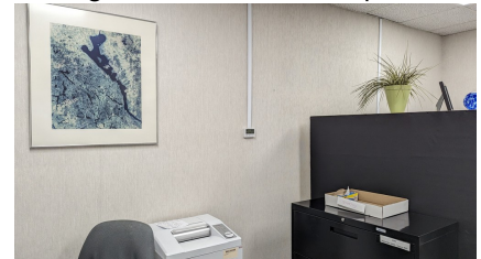
Figure 29: HRV controller in room 28
