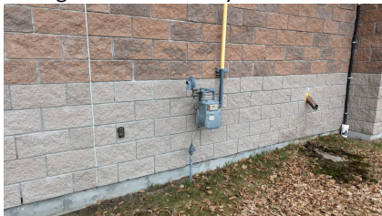
Figure 74: Natural gas meter - radio
