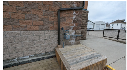
Figure 73: Natural gas meter - hall
