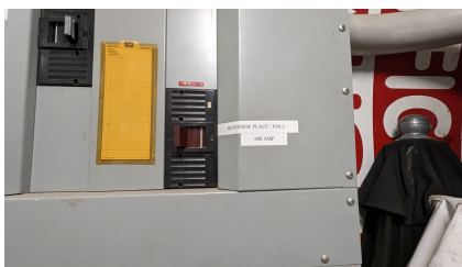
Figure 81: Main disconnect - hall
