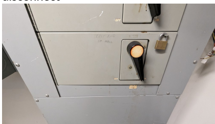
Figure 78: 200A disconnect for Panel D
