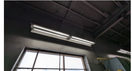
Figure 106: C - Type D - LED retrofitted fixtures
