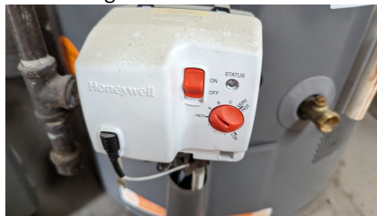
Figure 87: B - DHW03 - setting
