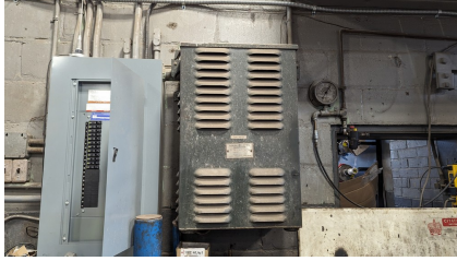
Figure 158: A - 15 kVA transformer
