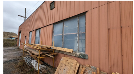
Figure 36: C - Windows in the water bay are in poor condition
