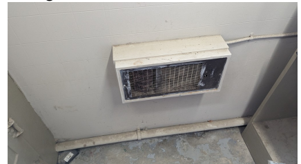
Figure 82: C - Electric heater in the women's washroom
