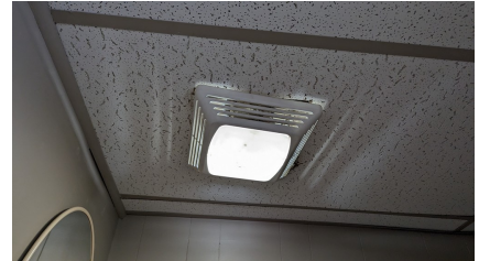
Figure 91: A - Type A - light and exhaust fan
