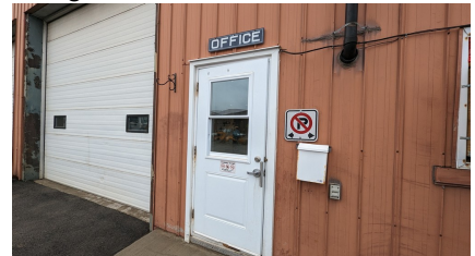
Figure 24: A - SE entrance door propped open by deadbolt
