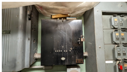
Figure 147: A - LDC meter cabinet
