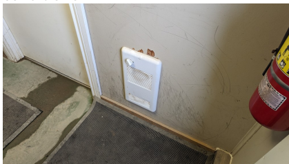
Figure 56: A - Electric cabinet heater in vestibule
