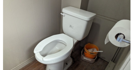
Figure 140: A - Toilet in the women's washroom
