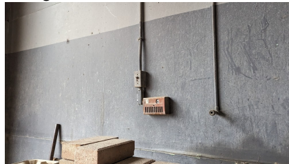
Figure 81: C - Old thermostat in the bay area
