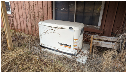
Figure 151: A - 11kW natural gas generator
