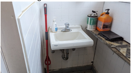
Figure 144: B - Handwashing faucet in washroom
