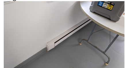
Figure 55: A - Lunchroom baseboard electric heater
