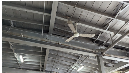
Figure 80: C - Ceiling fan in the bay area
