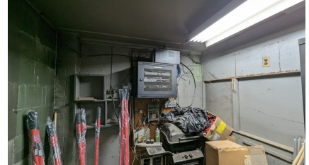
Figure 128: A - IT equipment in the former locker room
