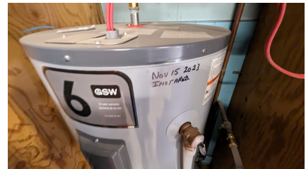
Figure 85: A - DHW02 - install date
