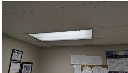
Figure 93: A - Type C - 2x4 fixture with fluorescent lamps
