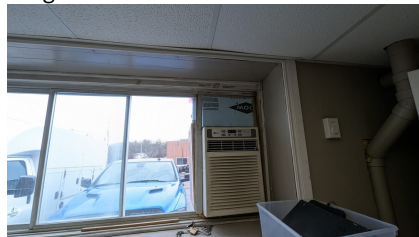
Figure 54: A - AC01 - front office air conditioner
