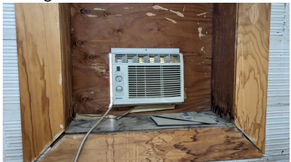
Figure 71: B - AC03 - window air conditioner
