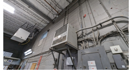
Figure 160: A - 45 kVA transformer in the bay area
