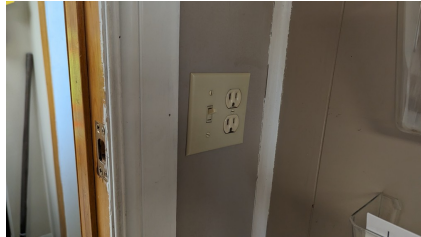
Figure 89: A - Manual switch in the office
