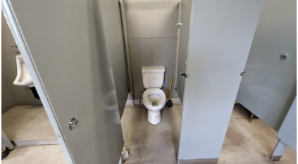
Figure 138: A - Toilet in the men's washroom
