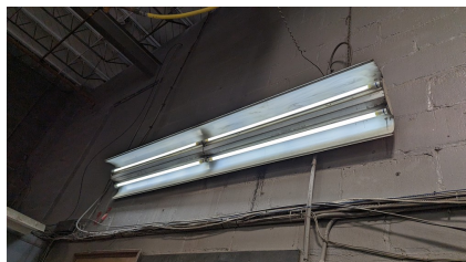
Figure 95: A - Type D - LED retrofitted fixtures
