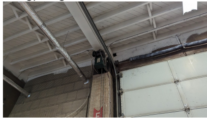
Figure 130: B - Garage opener
