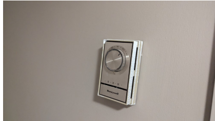
Figure 60: A - Wall thermostat in the women's washroom
