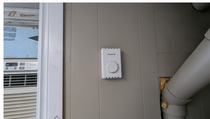
Figure 57: A - Thermostat controlling electric heater
