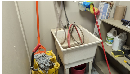
Figure 133: A - Laundry sink
