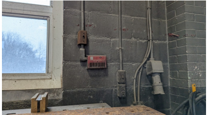
Figure 59: A - Old thermostat for a former unit heater
