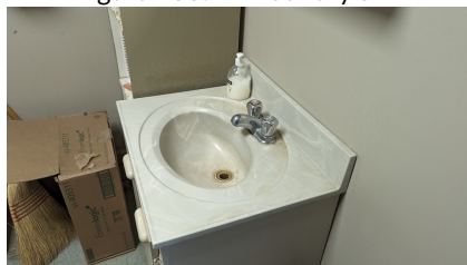
Figure 136: A - Lunchroom washroom faucet
