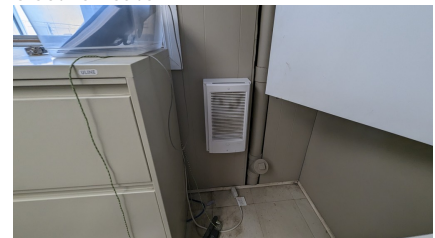
Figure 58: A - Electric cabinet heater in the front office
