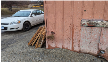
Figure 32: C - Damage to SE corner
