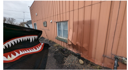
Figure 33: C - Damage on the north elevation
