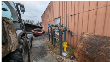
Figure 150: C - Natural gas meter
