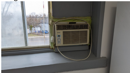
Figure 53: A - AC02 - lunchroom air conditioner
