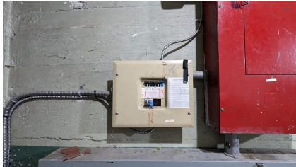
Figure 180: Panel B (boiler room)
