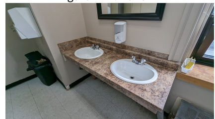
Figure 150: Handwashing faucets in the women's washroom
