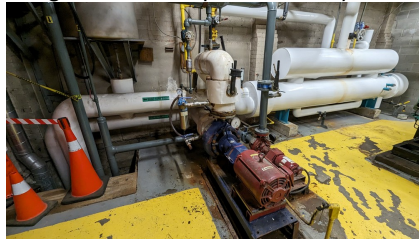
Figure 116: CP1 - cooling brine pump
