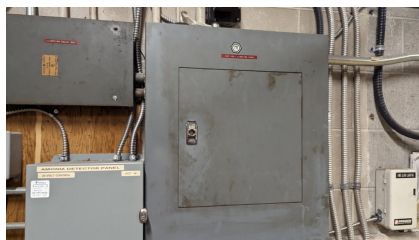
Figure 175: Lighting panel in ice plant room
