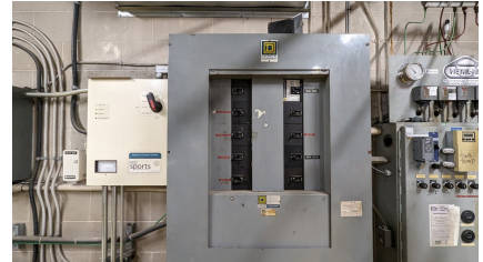
Figure 182: Panel in the ice plant room
