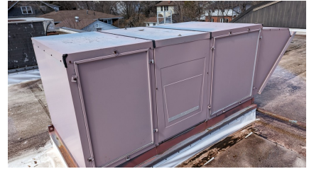
Figure 76: RTU no longer in use
