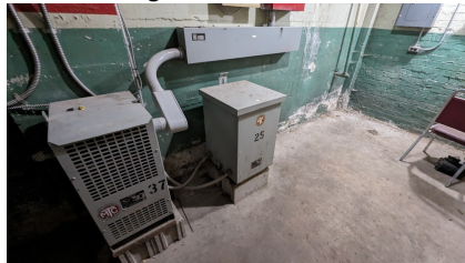
Figure 184: T25 - in boiler room
