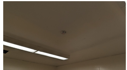
Figure 93: Occupancy sensor in dressing room 1
