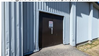
Figure 19: Hollow metal doors to ice rink
