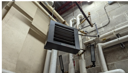
Figure 81: UH4 - mechanical room
