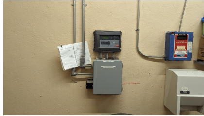
Figure 57: Gas detector controlling SSF1,2 and REF1,2
