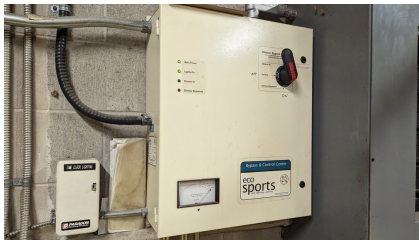
Figure 91: Light controls in the ice plant room
