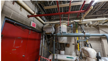
Figure 115: Brine expansion tanks
