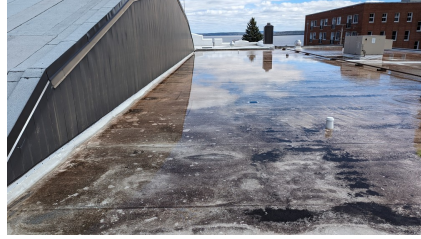
Figure 25: Standing water on the roof due to plugged CB
