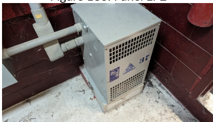
Figure 186: T37 - in electrical room
