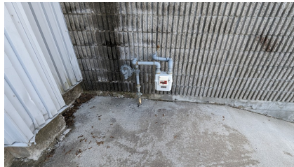
Figure 168: Natural gas meter on the north elevation
