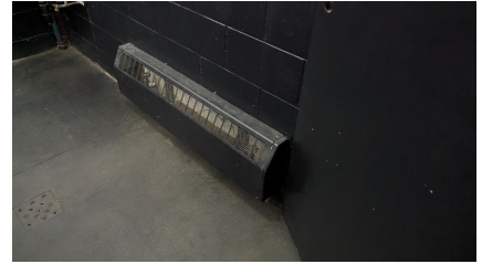
Figure 58: Hydronic baseboard heater in the referee changeroom
