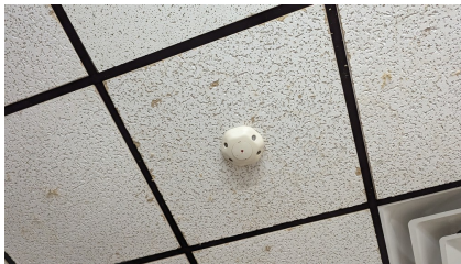
Figure 94: Occupancy sensor in men's washroom on first floor
