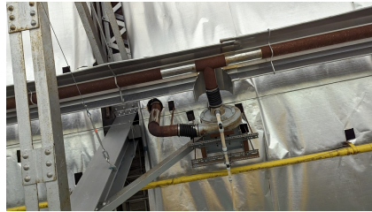
Figure 60: Infrared heaters in stands are in poor condition
