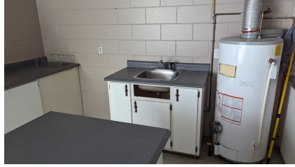
Figure 152: Kitchen sink in banquet kitchen
