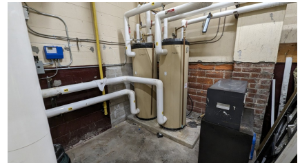
Figure 89: DHW3 and DHW4
