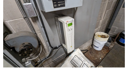
Figure 144: VFD for condenser fan
