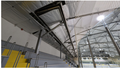
Figure 59: Infrared heaters over stands
