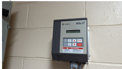
Figure 63: MUA1 - VFD appears to not be working
