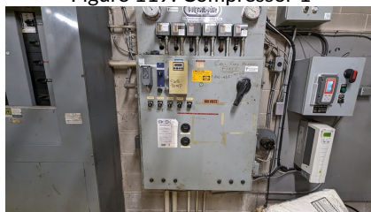
Figure 122: Control panel for ice plant
