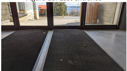
Figure 18: Gap present at bottom of main entrance door
