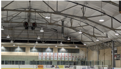
Figure 83: UH6 - gas-fired unit heater in area no longer used
