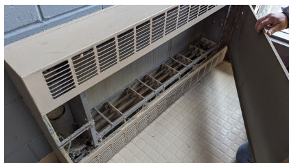
Figure 53: Electric cabinet heater in southwest stairwell
