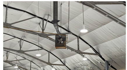
Figure 82: UH5 - gas-fired unit heater in area no longer used
