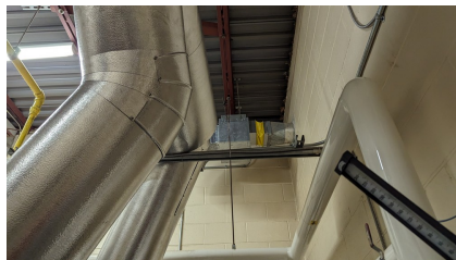
Figure 45: EF08 - DHW mechanical room
