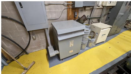
Figure 171: 75 kVA transformer in ice plant room
