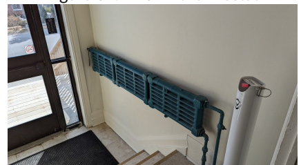
Figure 70: Radiator in east entrance
