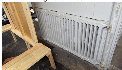
Figure 72: Radiator in 54s Changeroom
