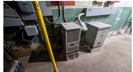
Figure 185: T37 - in boiler room
