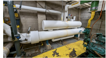
Figure 132: Ice plant chiller and surge drum
