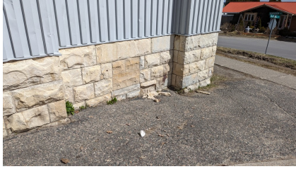
Figure 24: Spalling of the foundation
