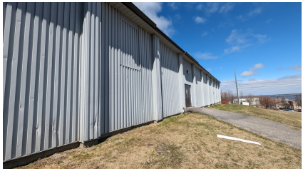
Figure 12: Damage to metal siding on east elevation
