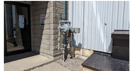
Figure 169: Natural gas meter on the south elevation
