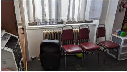
Figure 74: Radiator in the figure skating coach's room
