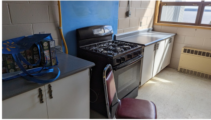
Figure 127: Gas stove in the banquet kitchen
