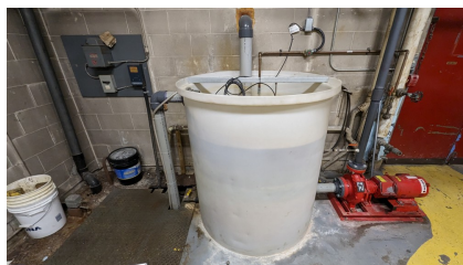
Figure 125: Evaporative condenser water tank
