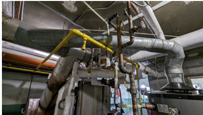
Figure 90: Missing insulation on DHW pipe
