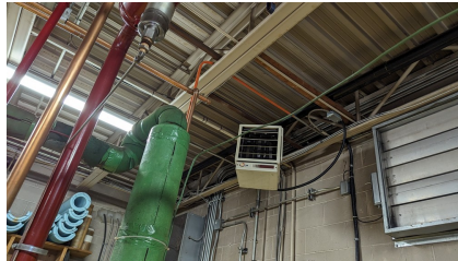
Figure 84: UH7 - electric - ice plant room
