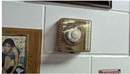
Figure 78: Thermostat in main lobby no longer used
