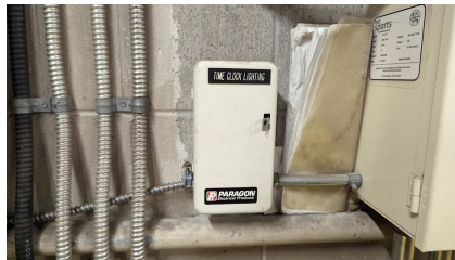
Figure 95: Time clock for arena lighting
