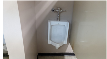
Figure 162: Urinal - 2nd floor washrooms
