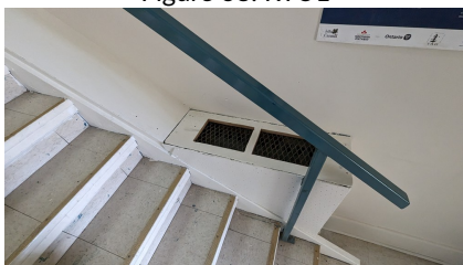
Figure 71: Radiator in the stairwell
