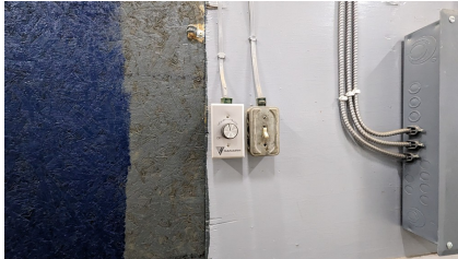
Figure 19: Ceiling fan control
