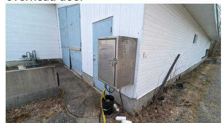
Figure 47: Fuel station control panel
