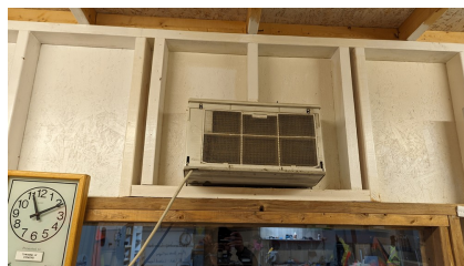
Figure 29: Unitary air conditioner with condenser faced out to shop area (AC1)
