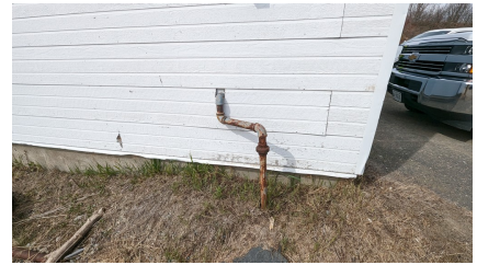
Figure 60: Natural gas piping that is going to UH1
