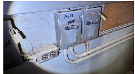
Figure 63: Fuel pump and washroom heater disconnects
