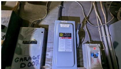
Figure 61: 60A disconnect for Panel LR
