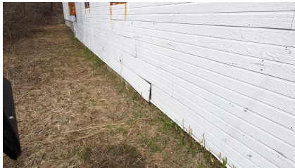
Figure 13: Siding is in poor condition
