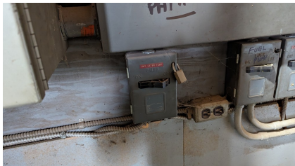
Figure 64: Hot water tank disconnect
