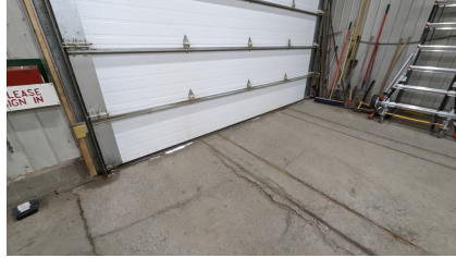
Figure 8: Gap at the bottom of the overhead door on the north elevation
