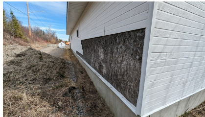
Figure 14: Siding missing on the cold storage side
