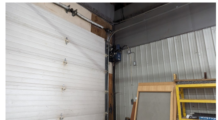
Figure 44: Door opener for the south overhead door
