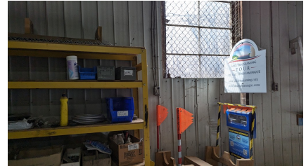
Figure 21: EF1 control switch
