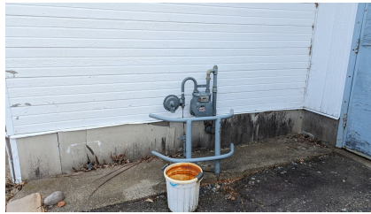
Figure 59: Natural gas meter
