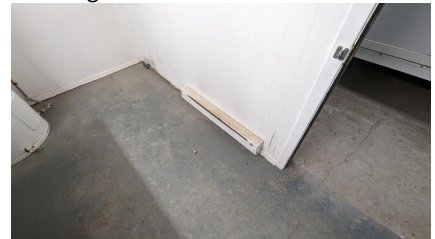
Figure 24: Electric baseboard in the washroom
