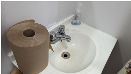
Figure 86: Handwashing faucet - office washroom
