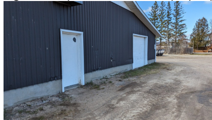
Figure 8: Damaged metal siding on the east elevation
