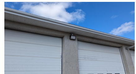
Figure 64: Type M - flood light with photocell
