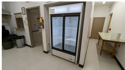
Figure 69: Cooler in kitchen
