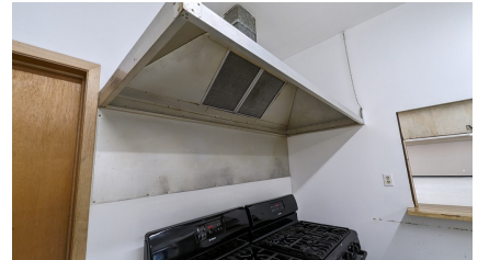
Figure 32: Range hood in the kitchen
