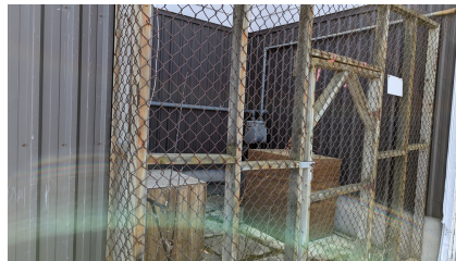
Figure 98: Natural gas meter
