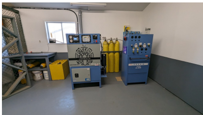
Figure 68: Breathable air compressors
