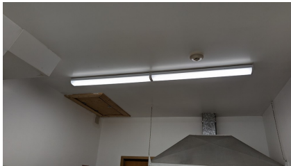
Figure 47: Type A - located in the kitchen
