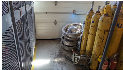
Figure 5: Bay 1 door not sealed properly
