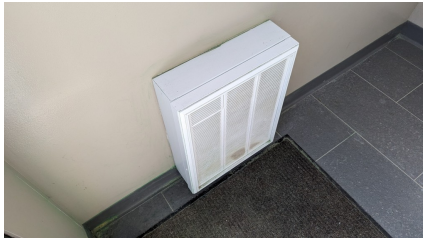
Figure 24: Electric heater in the community hall vestibule
