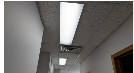
Figure 49: Type C - 1x4 fixture in office hallway
