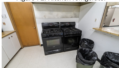
Figure 75: Natural gas stoves
