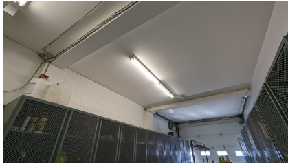
Figure 56: Type E - 2-lamp T8 strip fixtures
