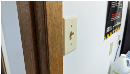
Figure 44: Manual light switch
