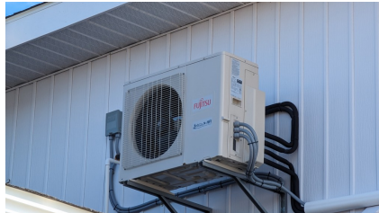
Figure 31: Mini split for the apartment
