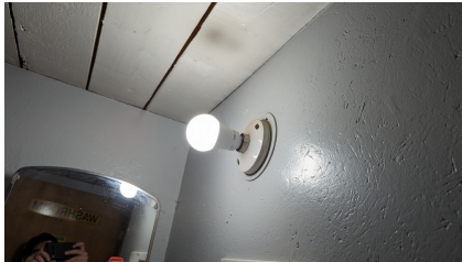
Figure 59: Type H - washroom LED lamp
