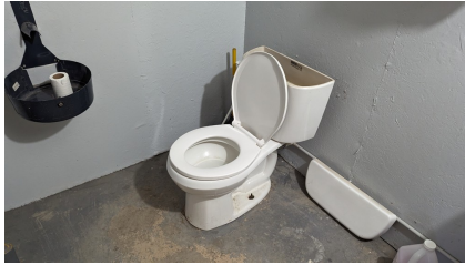
Figure 89: Public works toilet
