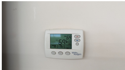
Figure 28: Fire training thermostat for electric baseboard heaters
