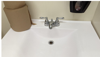
Figure 84: Faucet in second floor washroom
