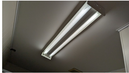
Figure 60: Type I - T8 lamps in upstairs washroom
