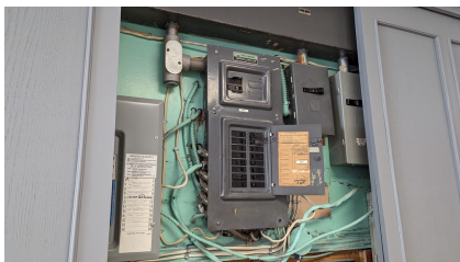
Figure 99: Generator Panel and Panel B
