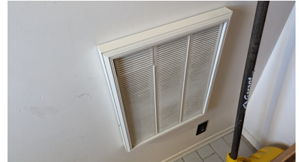
Figure 23: Electric heater in main entrance
