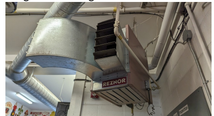
Figure 35: UH1 (recently replaced)
