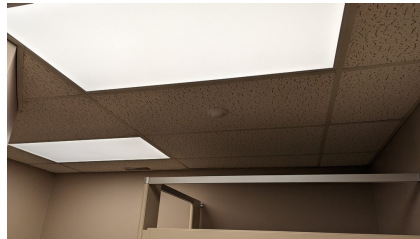
Figure 45: Occupancy sensor in men's washroom
