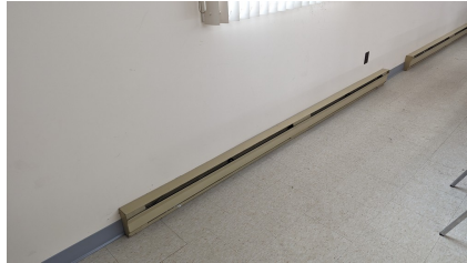
Figure 22: Electric baseboards in fire training room
