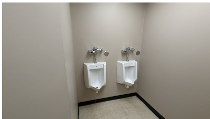
Figure 95: Urinals in men's washroom
