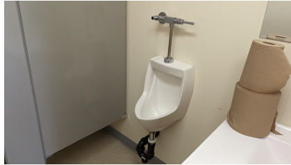
Figure 93: Urinal in second floor washroom
