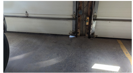
Figure 6: Bay 5 not properly sealing
