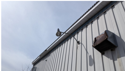
Figure 45: Old exterior fixture assumed to not be working
