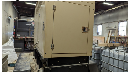
Figure 62: Portable generator in storage
