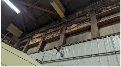
Figure 7: Damaged insulation in the mechanic bay
