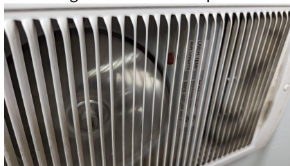
Figure 27: Electric cabinet heater in lunch room nameplate
