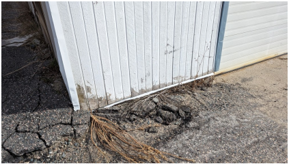
Figure 22: Wood siding deteriorating
