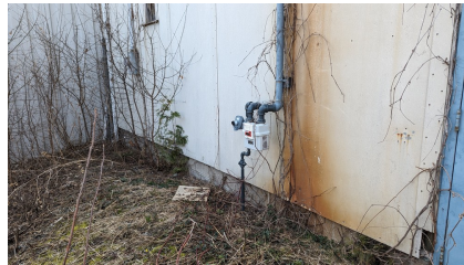
Figure 74: Natural gas meter
