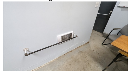
Figure 28: Electric cabinet heater in lunch room
