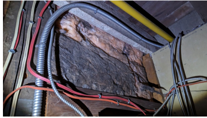
Figure 5: Batt insulation has mould on it
