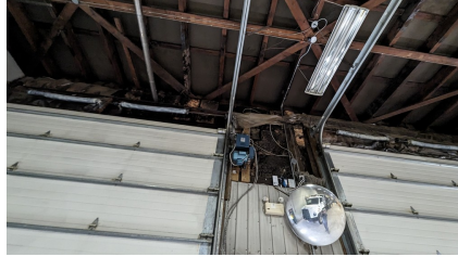
Figure 8: More damaged insulation
