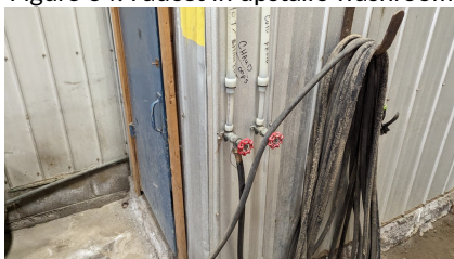
Figure 67: Hose bibs with hot and cold water supply
