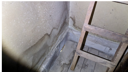
Figure 11: Gap in floor to the outside in the electric room
