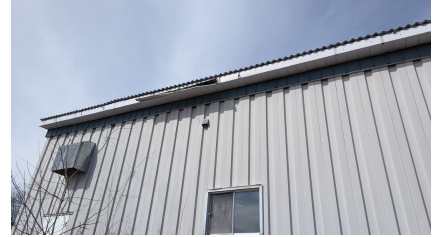
Figure 9: Eavestrough is missing
