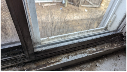
Figure 19: Window frame in poor condition
