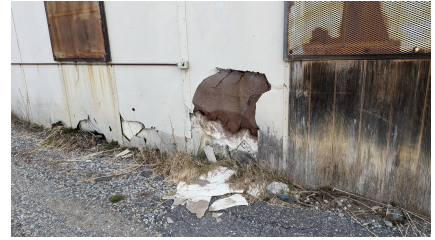
Figure 6: Damage to wall west elevation
