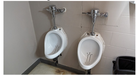
Figure 145: Urinals in 2nd floor washroom
