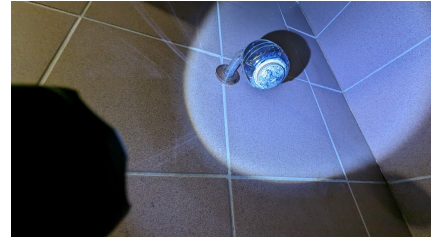
Figure 139: Showerhead in changeroom no 8
