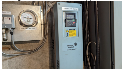
Figure 128: VFD for the evaporative condenser fan
