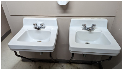
Figure 131: 2nd-floor washroom faucets
