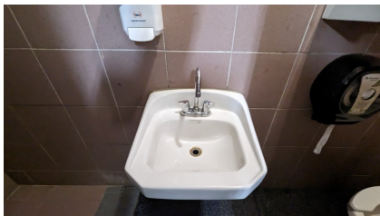
Figure 134: Handwashing faucet in changeroom no 8
