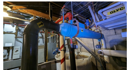
Figure 126: Subfloor heat exchanger
