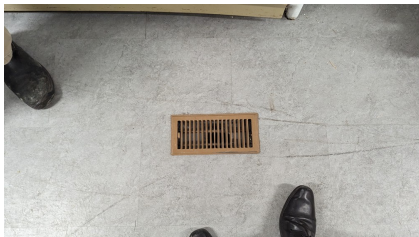
Figure 59: Supply register to the press room
