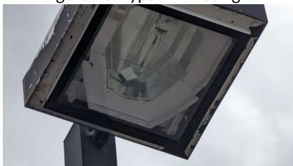
Figure 99: Type U - Parking pole lights
