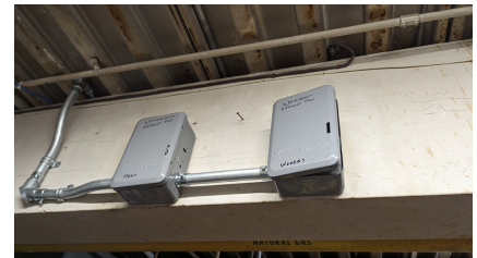
Figure 61: Timer for men's and women's washroom exhaust fan
