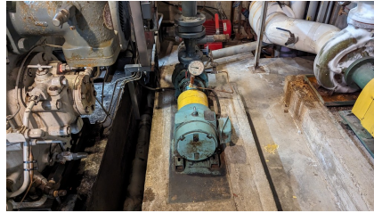
Figure 119: P02 - subfloor glycol
