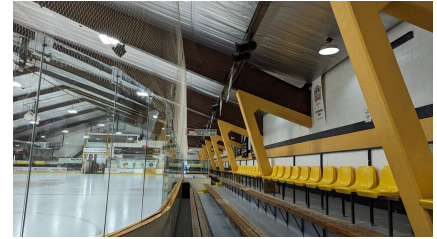
Figure 55: No heating on the south bleachers
