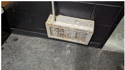
Figure 44: Electric heater in changeroom 5
