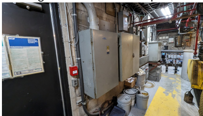
Figure 154: Main disconnect and electricity meter cabinet
