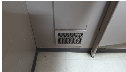
Figure 45: Electric heater in 2nd floor washroom
