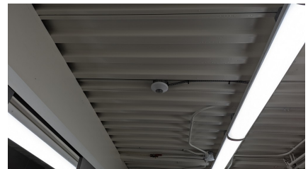
Figure 77: Occupancy sensor in the women's washroom
