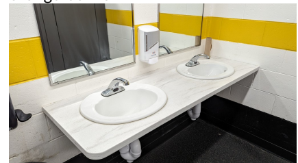
Figure 136: Low-flow handwashing faucets
