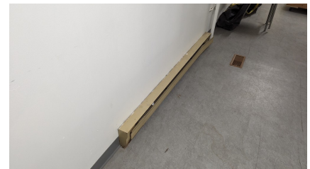
Figure 43: Electric baseboard heater in the press room
