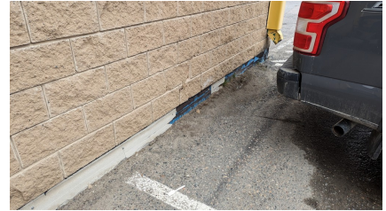
Figure 9: Damage to the south-facing wall
