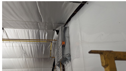
Figure 60: Supply vents for the ice rink
