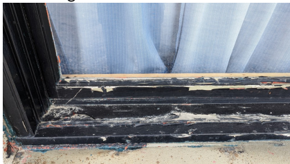
Figure 19: The office on the north elevation is in poor condition
