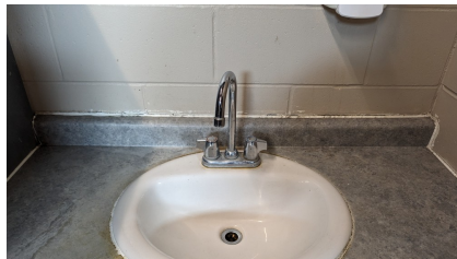
Figure 132: Handwashing faucet in changeroom 4
