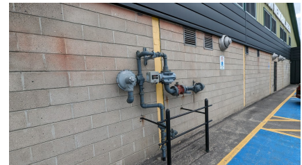
Figure 149: Natural gas meter
