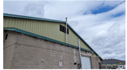
Figure 22: Air intake for the ice rink
