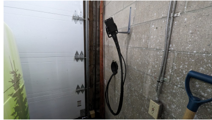
Figure 104: Charging station for ice resurfer
