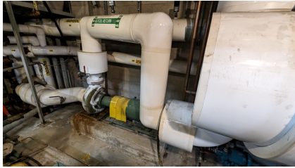
Figure 118: P01 - glycol cooling
