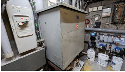
Figure 157: Transformer 1 - rated for 75 kVA
