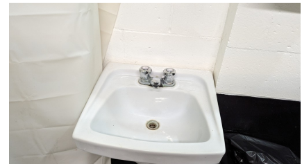
Figure 133: Handwashing faucet in changeroom 5
