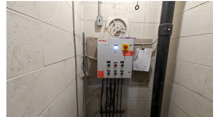
Figure 58: Sewage lift station
