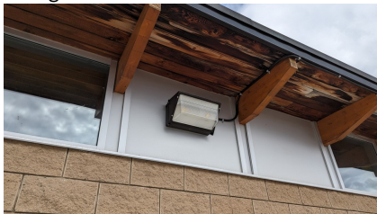
Figure 93: Type O - LED wall pack with photocell
