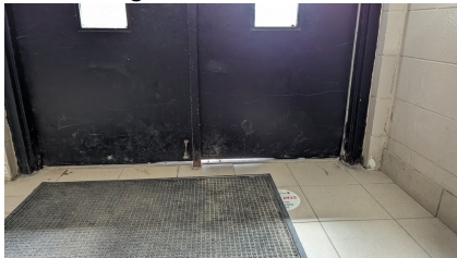
Figure 10: Door sweeps on the gymnastics entrance are in poor condition
