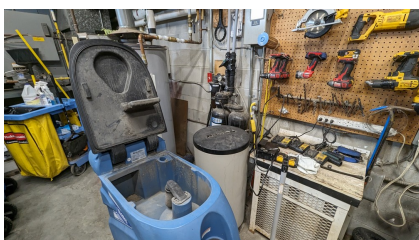
Figure 130: Water softener in the maintenance shop
