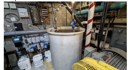
Figure 108: Cooling tower tank
