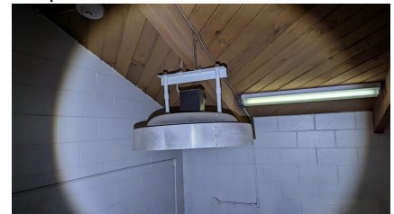
Figure 46: Electric heater in the former cloakroom
