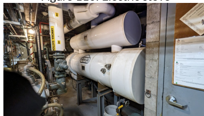
Figure 113: Ice plant chiller and surge drum
