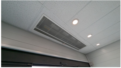
Figure 20: Air curtain in the main entrance
