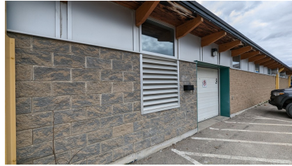
Figure 54: Intake louvre for F03
