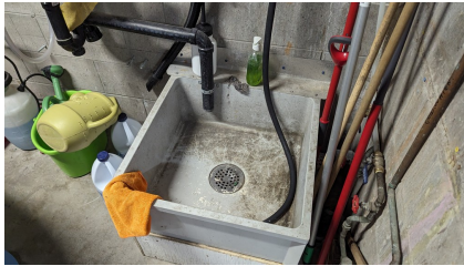
Figure 140: Slop sink in mechanical room
