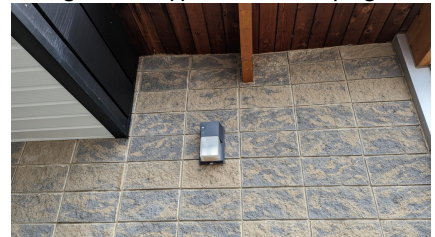
Figure 92: Type N - wall pack with photocell
