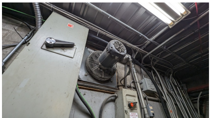
Figure 29: EF01 - ice plant room
