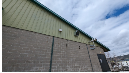
Figure 21: Air intake for DEH01
