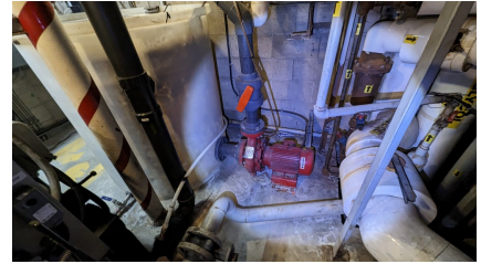
Figure 120: P03 - water spray pump
