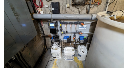
Figure 105: Chemical treatment for the evaporative condenser
