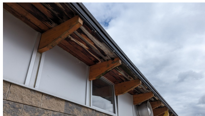
Figure 17: Soffit requires refinishing
