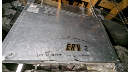
Figure 35: ERV2 is located in the ceiling space above the Storage room
