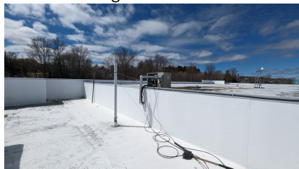
Figure 28: Ductless split unit
