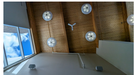
Figure 104: Type H1 fixtures in the lobby floor
