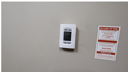
Figure 85: The thermostat in the boardroom
