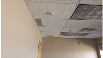
Figure 93: Ceiling-mounted occupancy sensor in the meeting room
