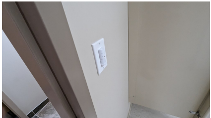
Figure 96: Switched-mounted occupancy sensor in the men's washroom
