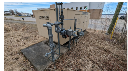
Figure 125: Natural gas meter serving the generator
