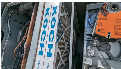
Figure 76: RTU3 filters are clean
