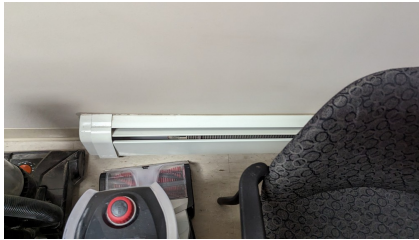
Figure 37: Electric baseboard heater in janitor closet
