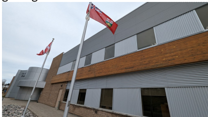
Figure 12: Laminated wood architectural feature in poor condition
