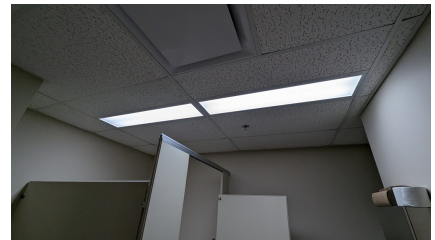
Figure 101: Type C fixtures in the men's washroom
