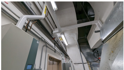
Figure 102: Type E fixture in the mechanical room
