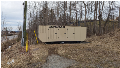
Figure 126: Natural gas generator
