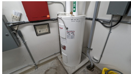
Figure 92: Electric DHW tank in the mechanical room
