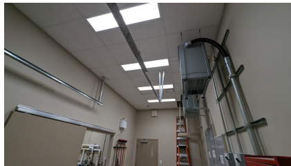
Figure 100: Type C fixtures in the receiver room
