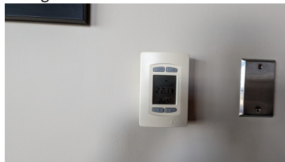
Figure 86: The thermostat in the council chambers
