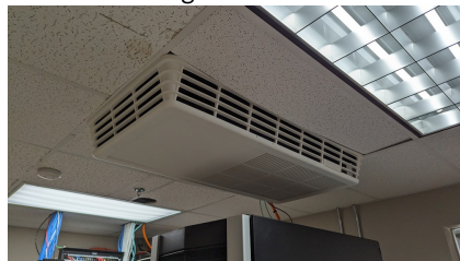
Figure 29: Ductless split unit in the IT room
