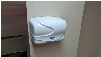
Figure 109: Electric air dryer in the men's washroom
