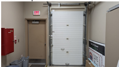
Figure 15: Overhead in the Receiver room
