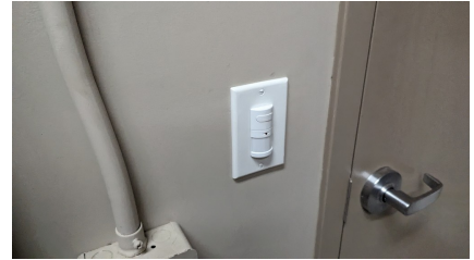
Figure 95: Switched-mounted occupancy sensor in the receiver room
