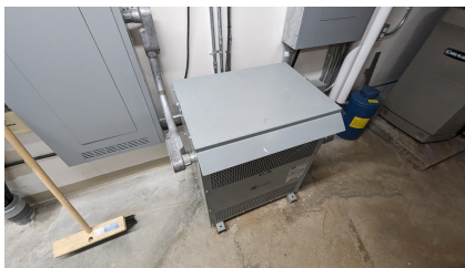
Figure 127: 75 kVA transformer to panel PP-A
