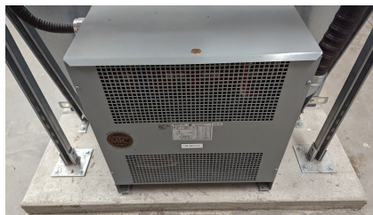
Figure 128: 75 kVA transformer for RTU1 and RTU2
