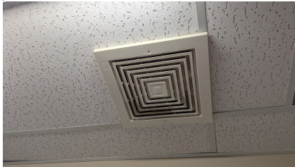
Figure 40: The exhaust fan is controlled via a thermostat in the elevator room
