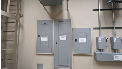
Figure 133: Panel IG-PC, B, and DP-2 in the Receiver room
