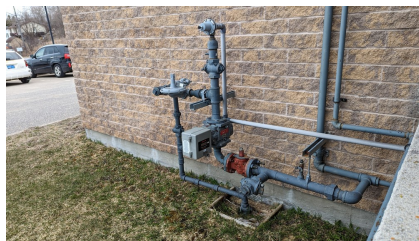
Figure 124: Natural gas meter for the building
