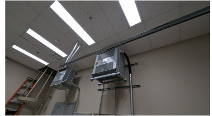
Figure 135: Two 45 kVA transformers in the Receiver room
