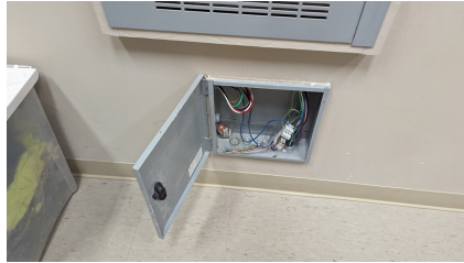
Figure 94: Contactor for northern parking lot lights that connect to the BAS
