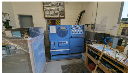
Figure 60: Breathable air compressor
