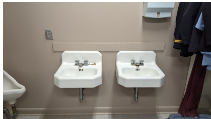
Figure 69: Faucets in the upstairs washroom
