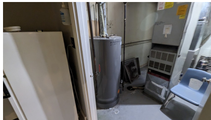
Figure 39: DHW tank in the mechanical room
