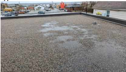
Figure 14: Pooling water on the roof above the firehall
