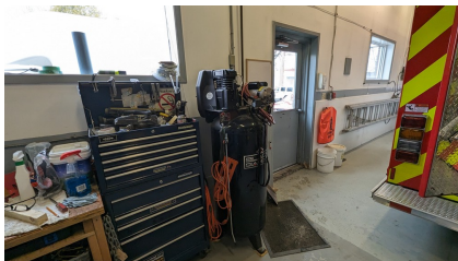
Figure 59: Air compressor in the firehall
