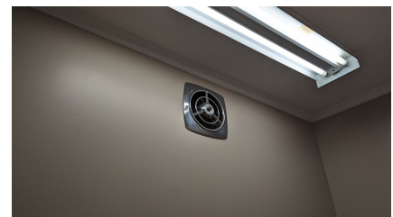
Figure 29: Exhaust fan in the upstairs washroom
