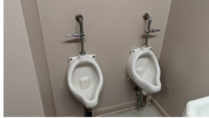
Figure 75: Urinals in the upstairs washroom
