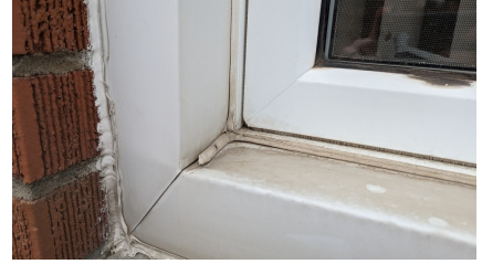
Figure 22: Window seal fail
