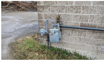
Figure 77: Natural gas meter
