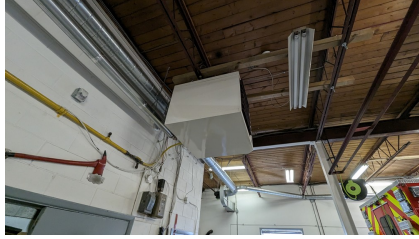
Figure 37: Unit heater in the firehall
