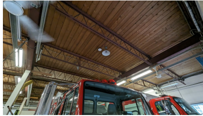
Figure 42: Original fixture no longer used
