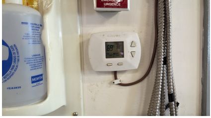
Figure 36: Thermostat controlling the unit heater in the firehall
