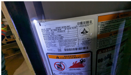
Figure 38: DHW tank information
