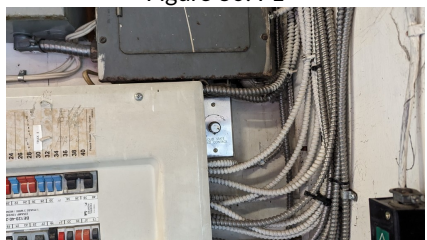
Figure 33: Fan control in the firehall
