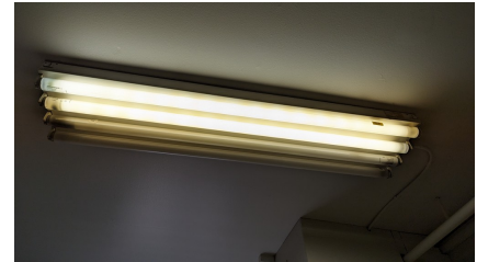
Figure 52: Type E - surface-mounted T12 fixture with magnetic ballast
