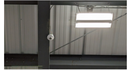
Figure 45: Occupancy sensor in the apparatus bay
