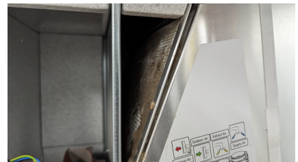
Figure 25: HRV1 dirty filter
