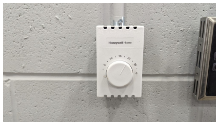
Figure 35: Thermostat controlling IH2
