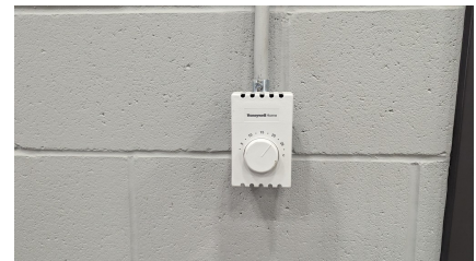
Figure 34: Thermostat controlling IH1
