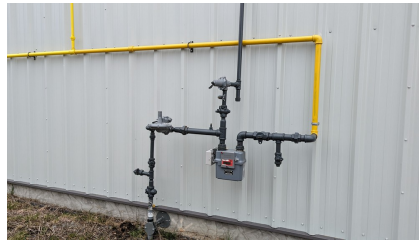
Figure 82: Natural gas meter
