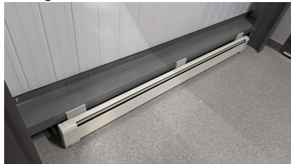
Figure 29: Hydronic baseboard heating in 2nd floor storage room
