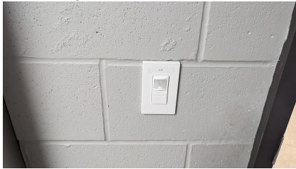
Figure 46: Switch-mounted occupancy sensor
