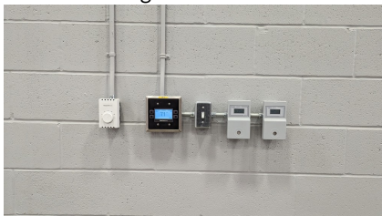
Figure 20: CO and NO2 sensors for MUA1 on the right
