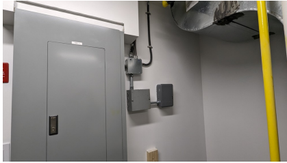
Figure 43: Astronomic control for exterior lights
