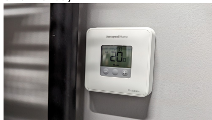
Figure 36: Thermostat for hydronic baseboard heating on 2nd floor
