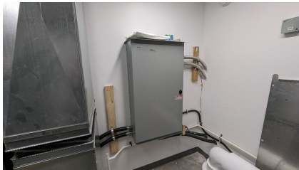
Figure 85: Automatic transfer switch
