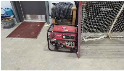
Figure 83: Back up portable generator
