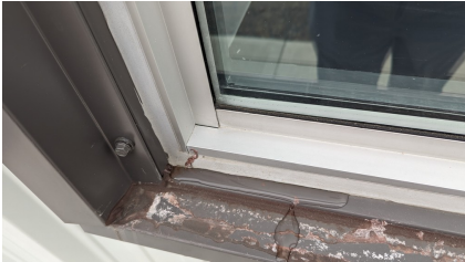
Figure 13: Window frame beginning to rust
